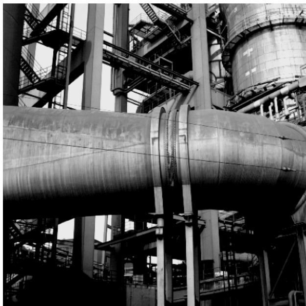
compensator in a pipe in of a blast-furnace
