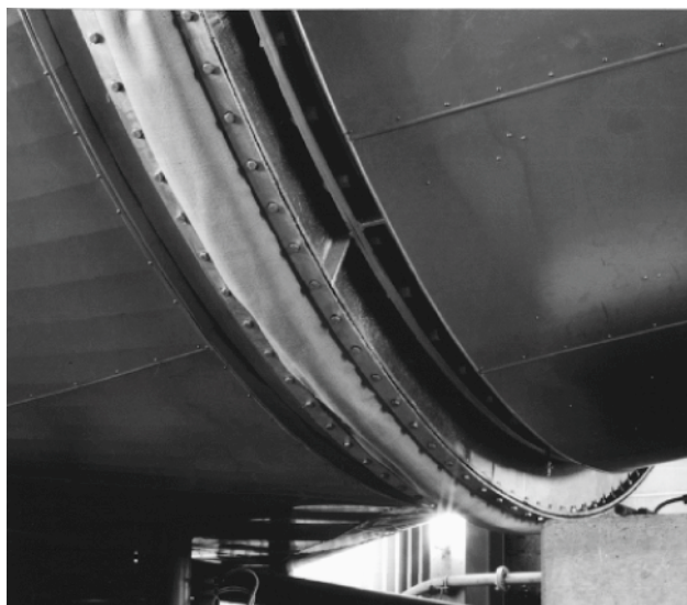
KLINGER Kempchen compensators in flue gas distributing main
