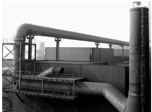
Compensators at the entrance to a heat recirculation pipe at a sintering plant
