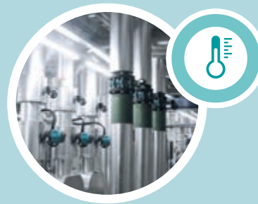
HVAC & Swimming Pools
